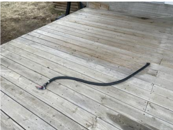
Bottom deck is wired for hot tub.
