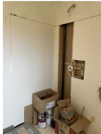
Plumbed for shower
