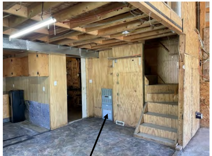
Main floor - propane furnace
