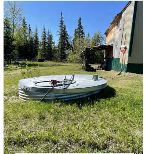
3000 gallon water cistern
