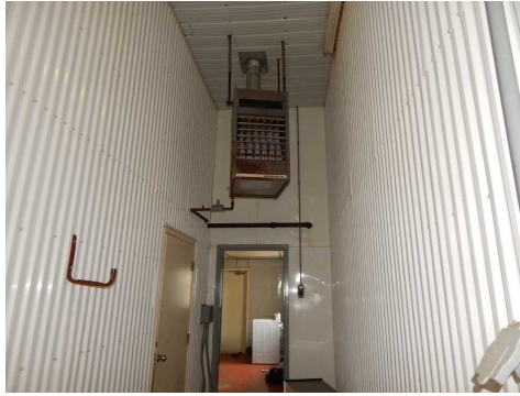
Furnace in hallway from former changing room
