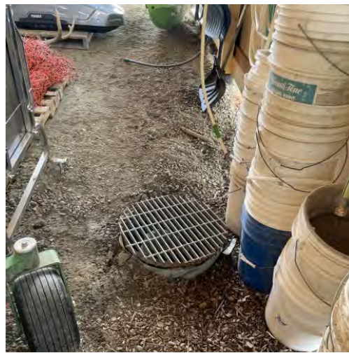
WATER WELL Located in north lean to on shop
